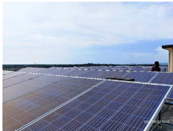
Solar Power plant
