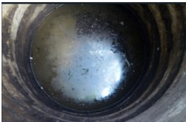
Well with Non potable water
